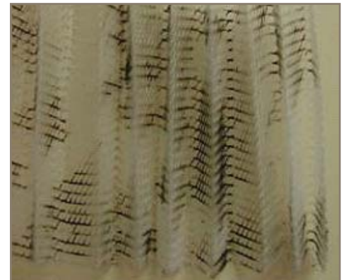
Burnt polymer pleat support mesh from arcing
